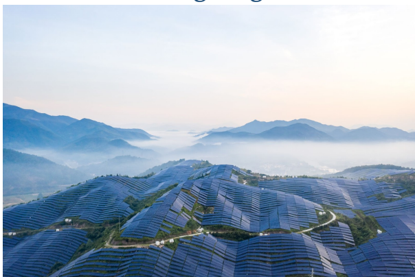
An aerial view of a solar power station in the mountains of Fujian, China. (Source: Getty Images, Royalty-Free)
